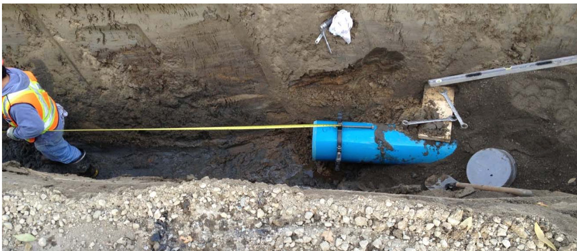
Infrastructure pipe. © RDOS
