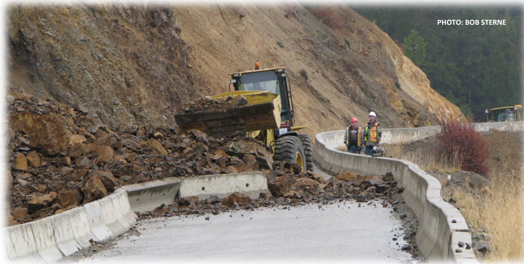
Rock Slide on Coalmont Road
