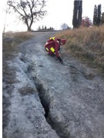
Photo 22 Subsurface erosion and deep cavity on access to KVR at Newton Road
