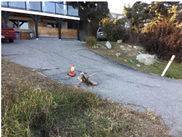
Photo 15 Small sinkhole in driveway (Sage Mesa)
