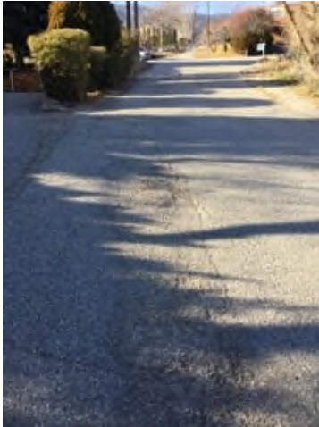
Photo 17 Depressions in road (end of Duchess Dr)
