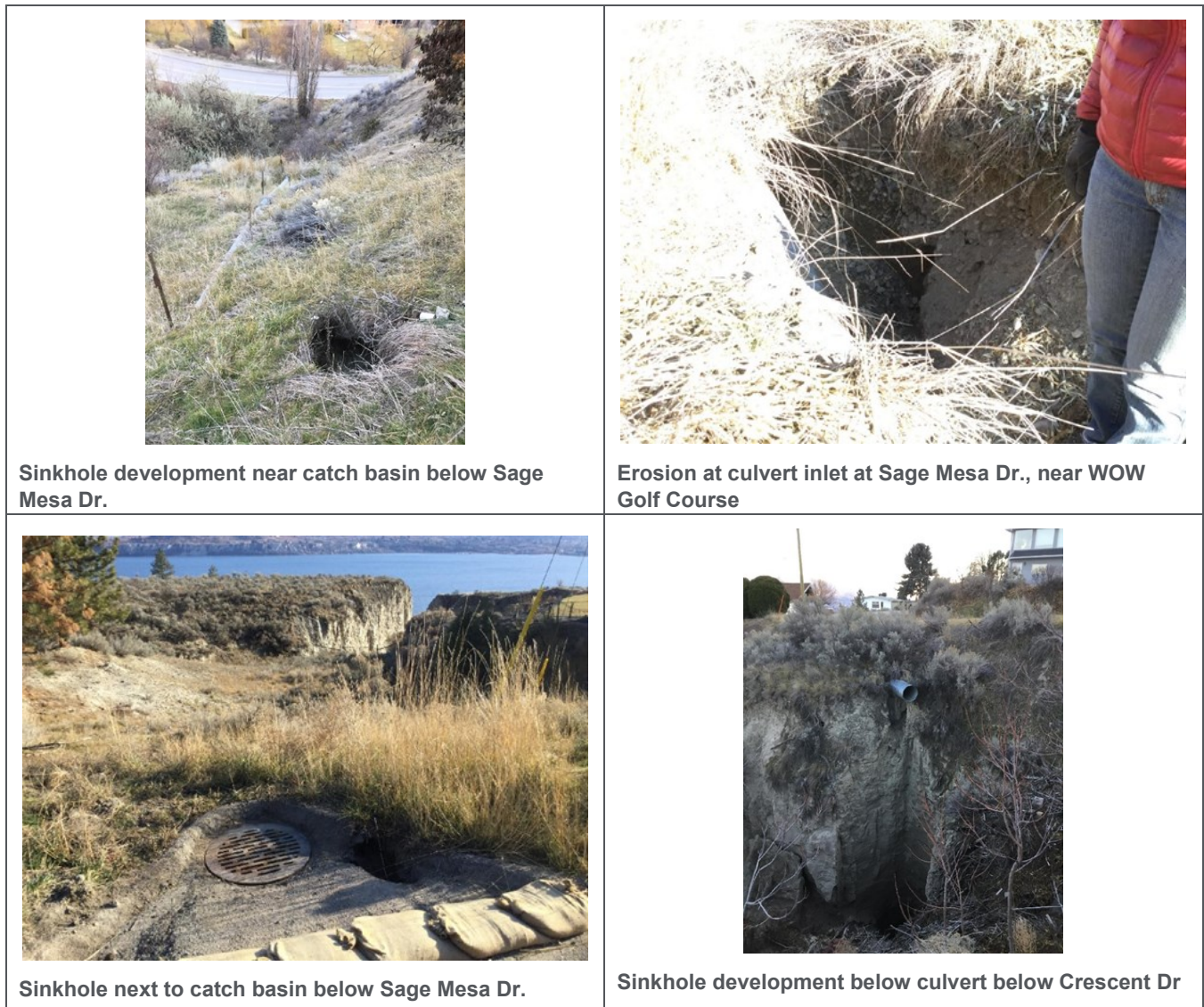
Figure 4.3.a Photographs of Example Sinkholes and Erosion Features Associated with Stormwater Management in the GWB Study Area
