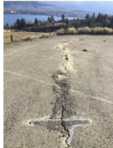
Photo 10 Pavement cracking at WOW GC
