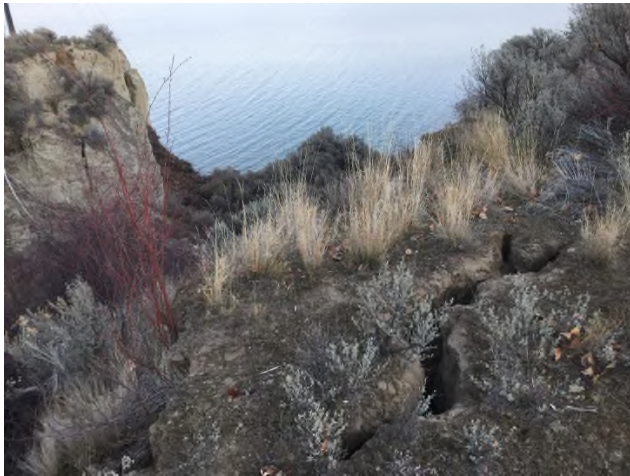
Photo 13 Tension crack at gully edge (Sage Mesa)
