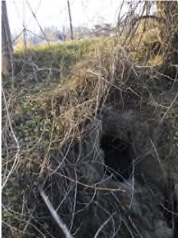
Photo 21 Sinkholes at gully crest (Newton Dr and Duchess Dr)
