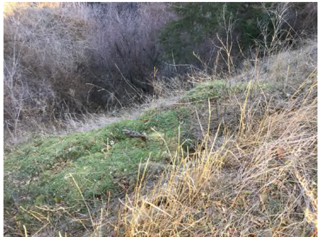
Photo 20 Tension cracks and landslide activity along crest of gully (Newton Dr and Duchess Dr.)
