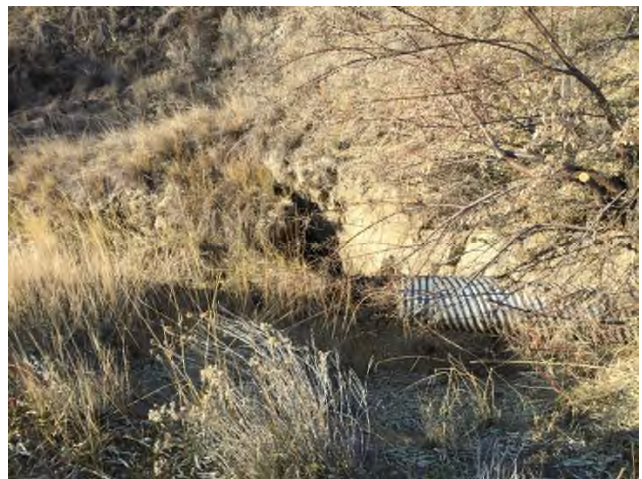
Photo 8 Erosion at culvert outlet at Sage Mesa Rd crossing (near WOW GC)
