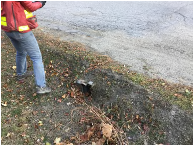
Photo 3 Damaged culvert inlet (Sage Mesa)
