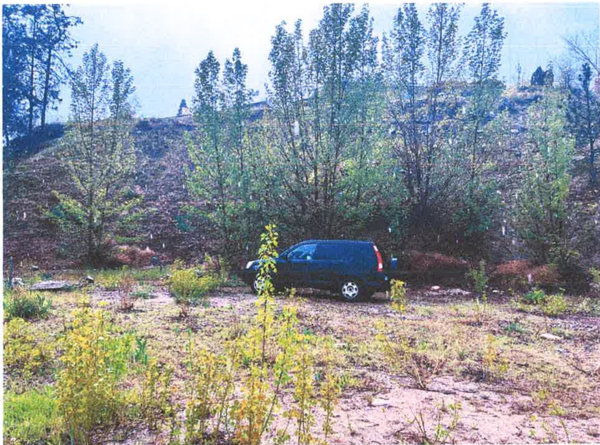
Photo No. 2 – Steep north slope. Note boulders on slope and at toe of slope
