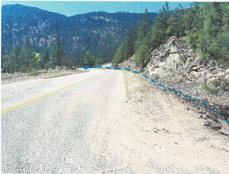
Photo No. 3 : View looking west down Forsyth Drive towards location where any pool leakage or runoff water would infiltrate into the soils along the ditch and eventually make its way to Madeline Lake. (2023 07 31). See attached Figure 3 – Drainage Route for approximate runoff path.
