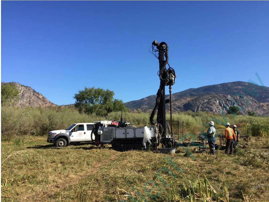
Photo 3: Drilling monitoring wells at the Site using a sonic drill rig (October 2, 2017).
