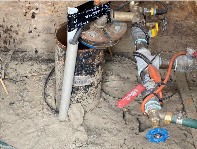
4. View of wellhead of WTN 105407 (WPID 27891) inside wooden well enclosure. Datalogger deployed inside white PVC stilling well during pumping test with WTN 124408. View looking north.
