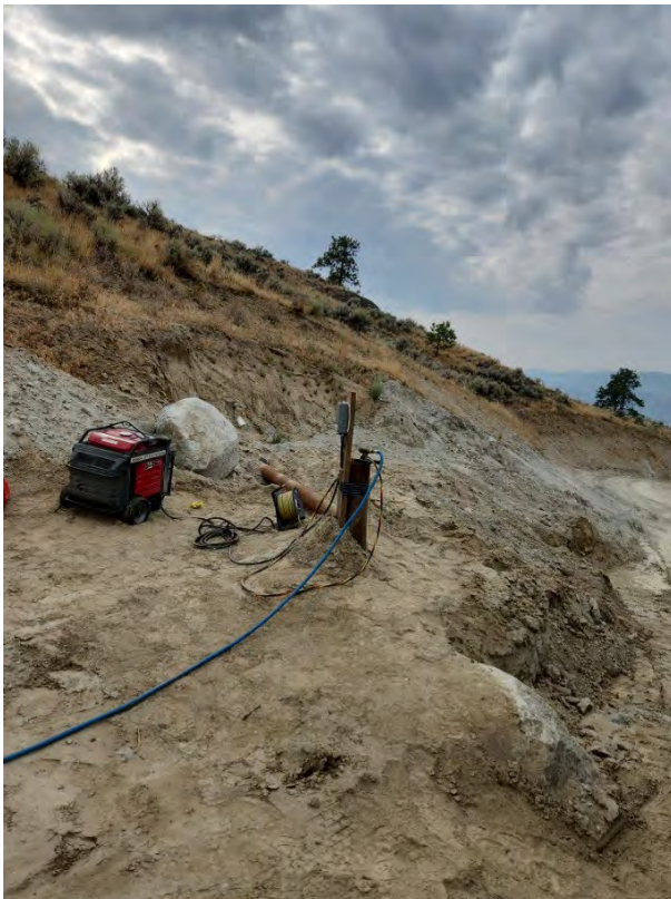
8. Pumping test on WTN 124408. Depiction of new casing stickup (nominally 0.6m above current ground elevation) to facilitate pumping test. View looking south.
