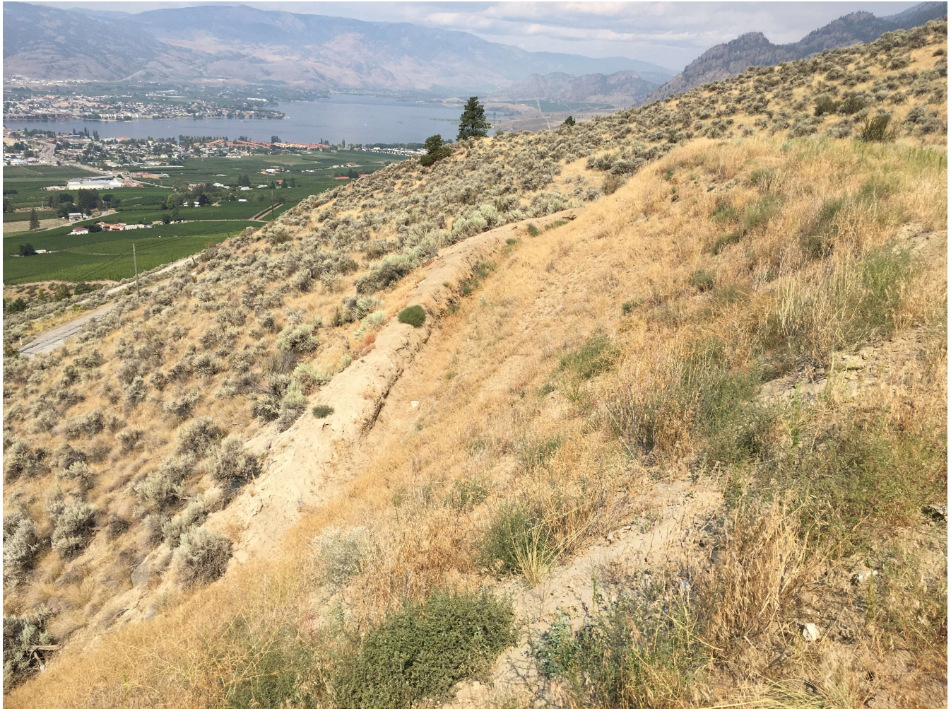
Photo 9 View of the north side and slope of the uncontrolled fill prior to the stockpiling of blast rock, looking north.
