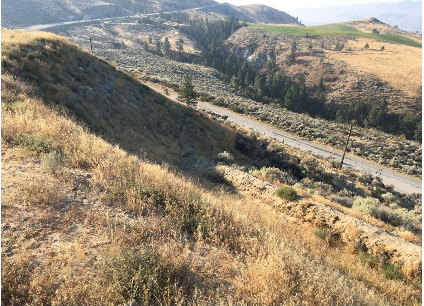
Photo 8 Downslope view from northwest crest of the uncontrolled fill, looking southwest. A berm to stop material from rolling towards Highway 3 is located at various points around the area, but not around the complete area of uncontrolled fill.
