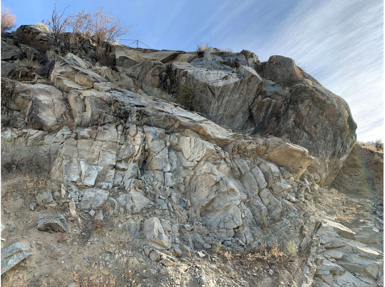
Photo 4 View of scaled and blasted bedrock east of the access road looking east. Rockfall mitigation can be seen at the top of the photo.
