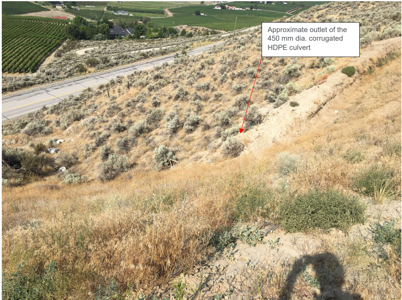
Photo 12 Approximate outlet location downslope of the toe, of the 450 mm corrugated HDPE culvert running below the uncontrolled fill. Highway 3 can be seen running northwest-southeast in the background, photo looking west.
