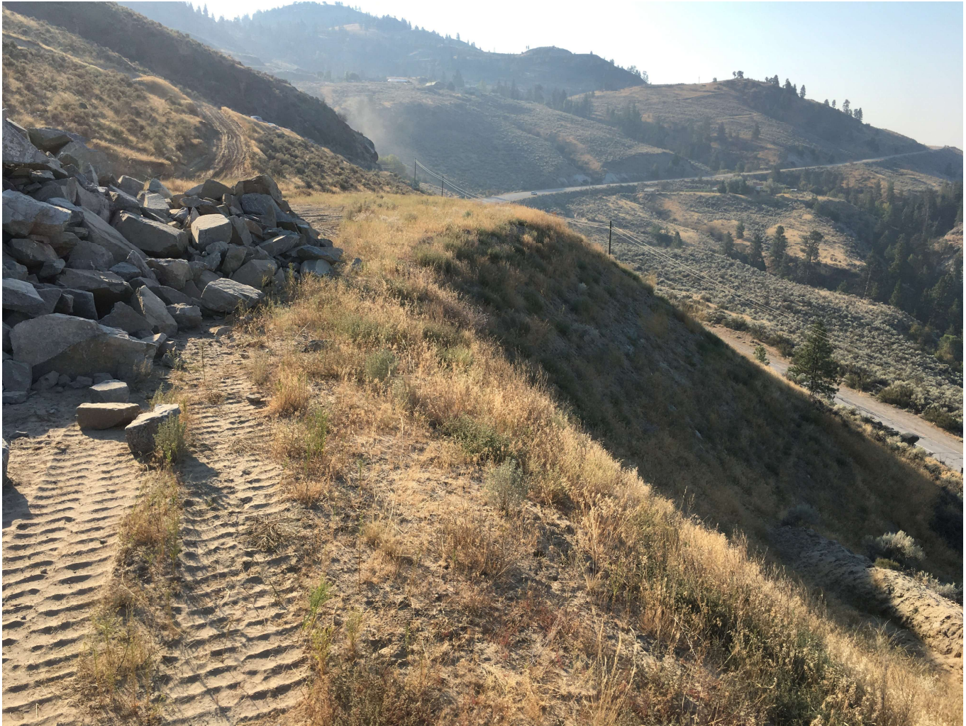
Photo 7 View of the uncontrolled fill, looking south. Blast rock is currently being stored in the area. The access road to the south portion of the fill can be seen in the top left corner of the photo.
