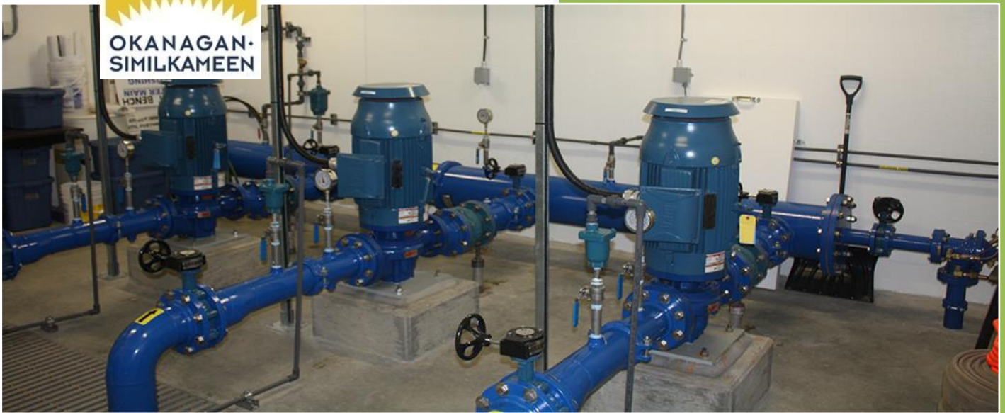
West Bench Booster Pump Station
