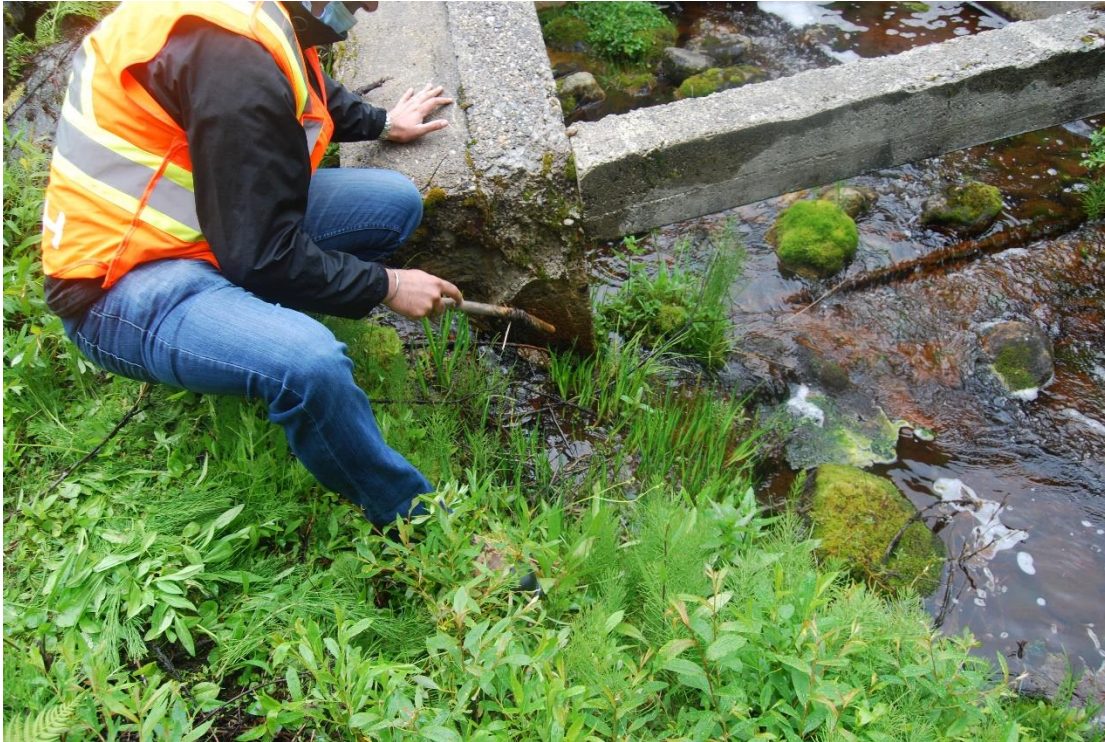
Photo A7: Big Meadow Lake Dam Outlet Works, Seepage from Right Wall Area
