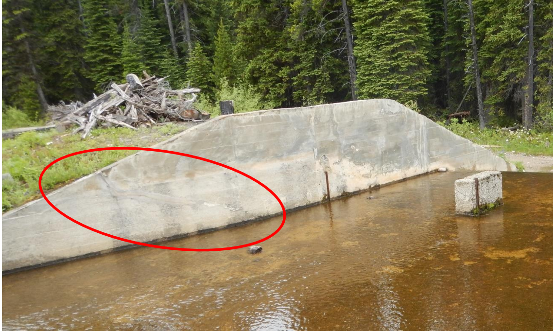
Photo A19: Big Meadow Lake Dam Spillway Repaired Crack in Left Retaining Wall
