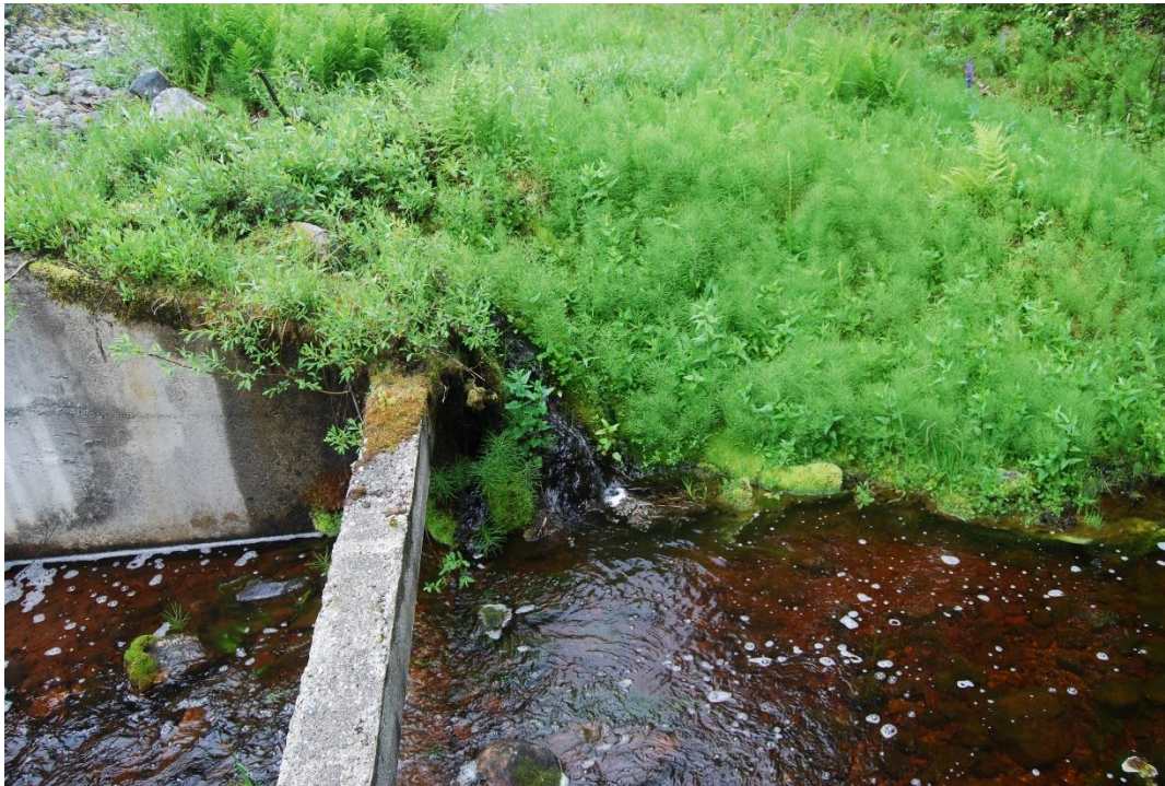
Photo A6: Big Meadow Lake Dam Outlet Works, Seepage from Left Wall Area
