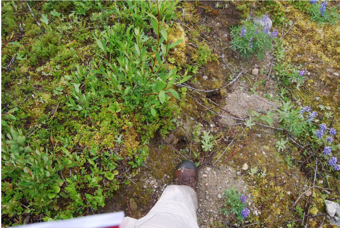
Photo A15: Big Meadow Lake Dam, Minor Animal Burrow on Dam Upstream Slope
