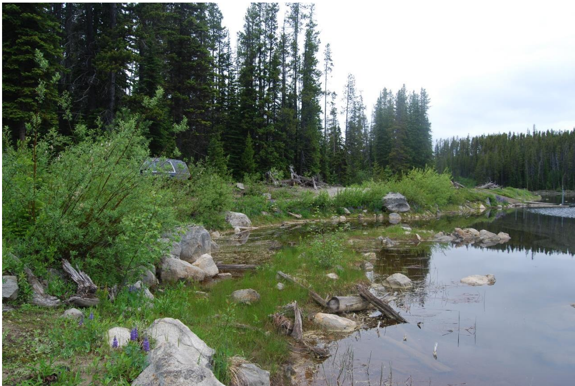
Photo A14: Big Meadow Lake Dam Upstream Slope close to Left Abutment
