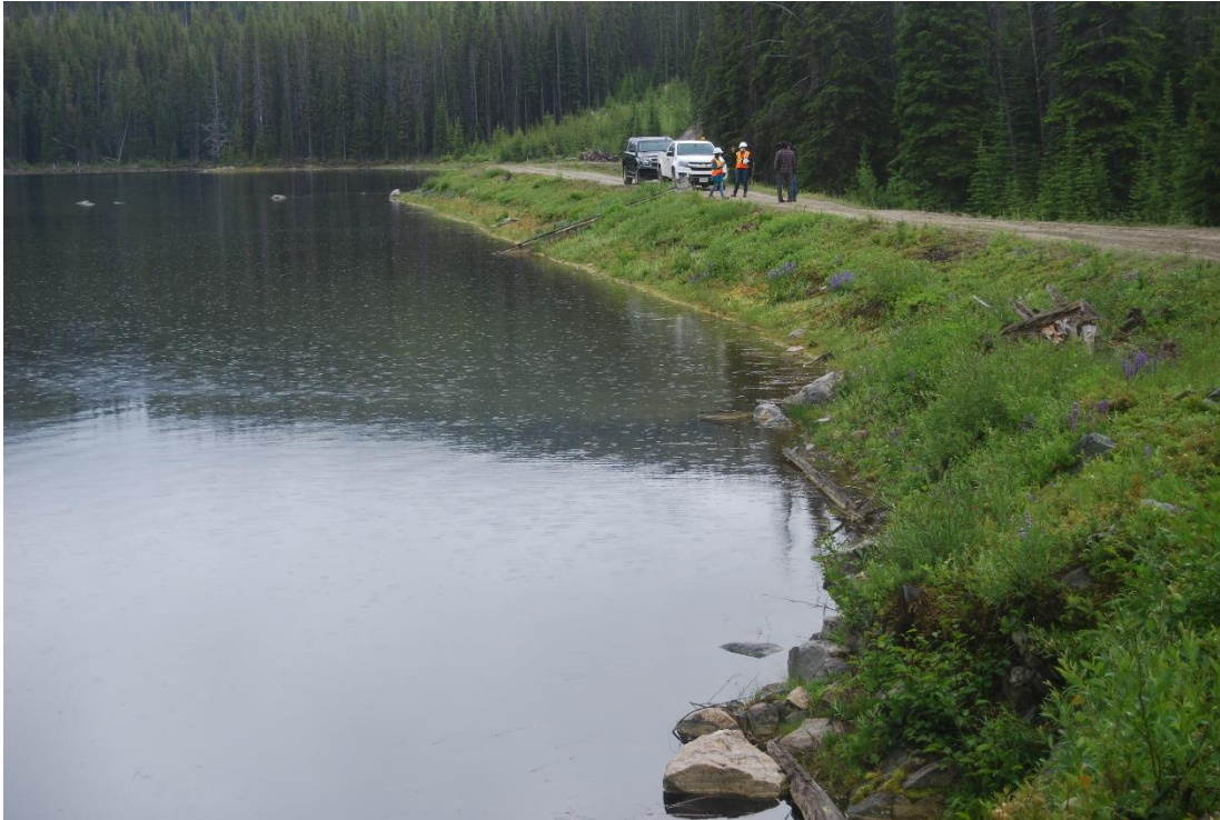
Photo A1: Big Meadow Lake Dam Upstream Slope, Looking from Right Abutment
