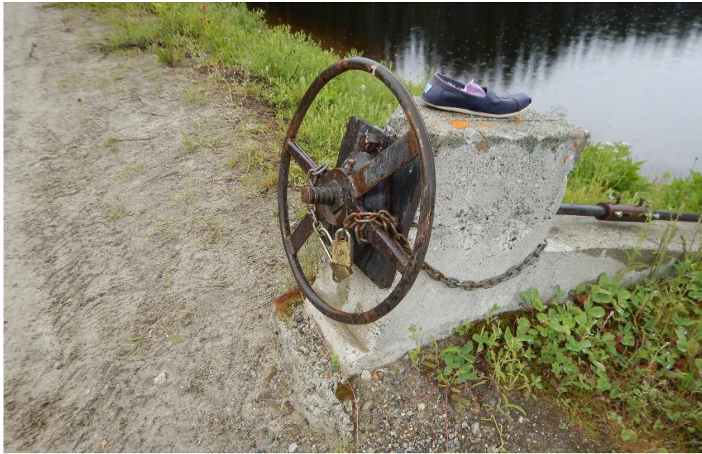
Photo A17: Big Meadow Lake Dam Intake Gate Operating Wheel Assembly
