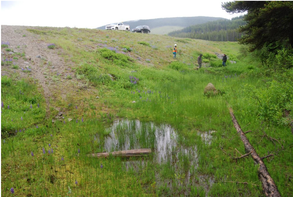
Photo A4: Big Meadow Lake Dam downstream slope, Looking at Outlet Works Location
