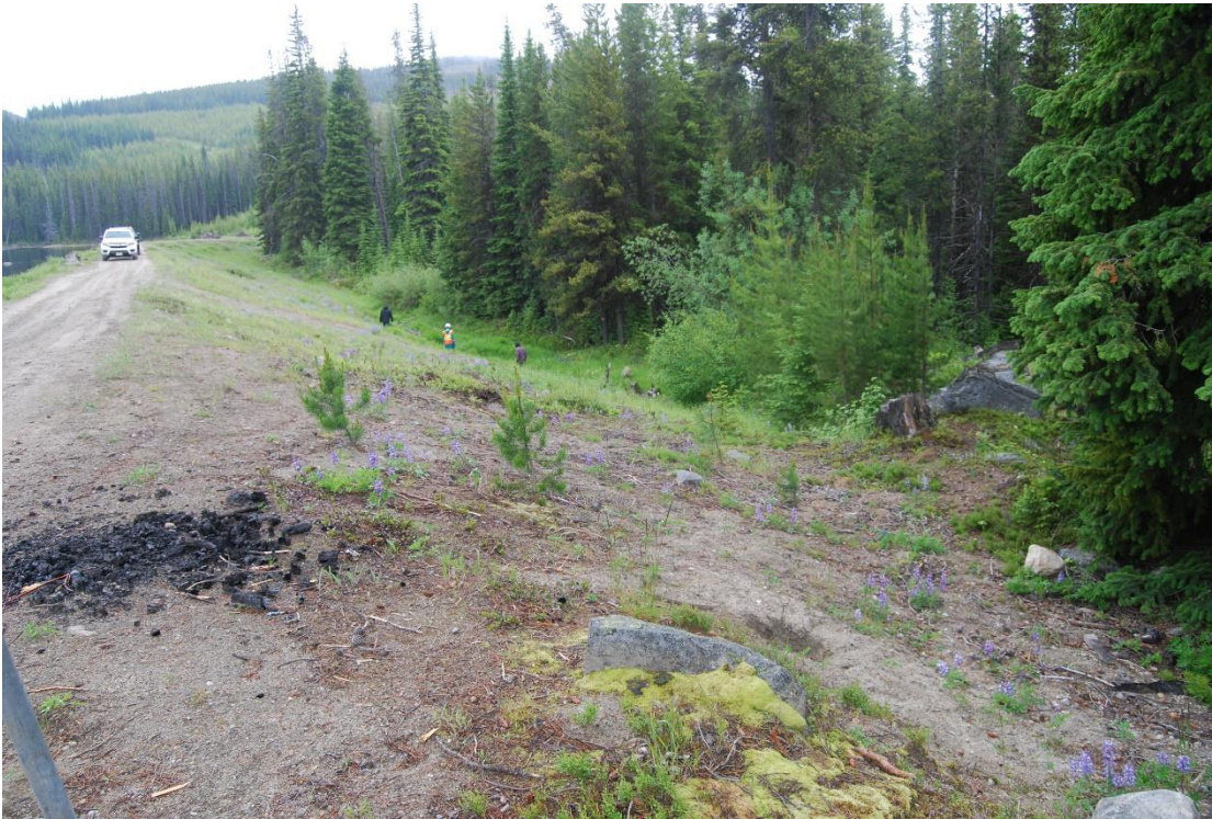
Photo A3: Big Meadow Lake Dam Downstream Slope, Looking from Right Abutment
