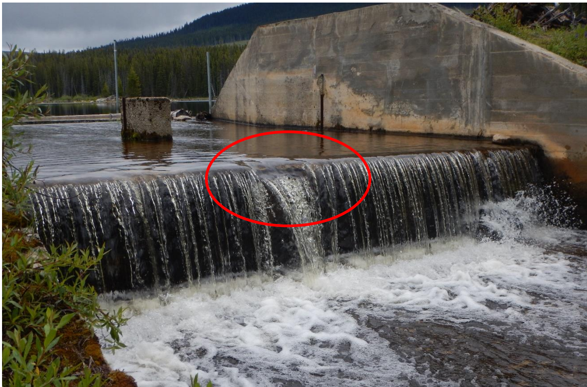
Photo A18: Big Meadow Lake Dam Spillway Crest Concrete Damage at Mid Span
