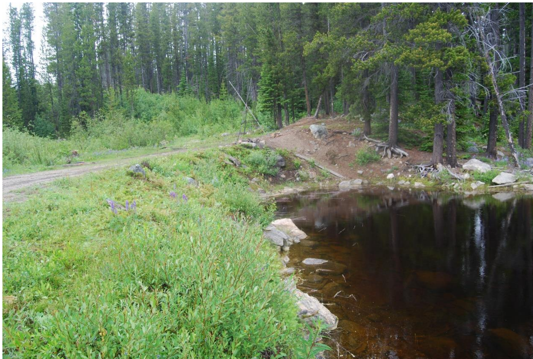
Photo A2: Big Meadow Lake Dam Crest, Looking at Right Abutment and Slope
