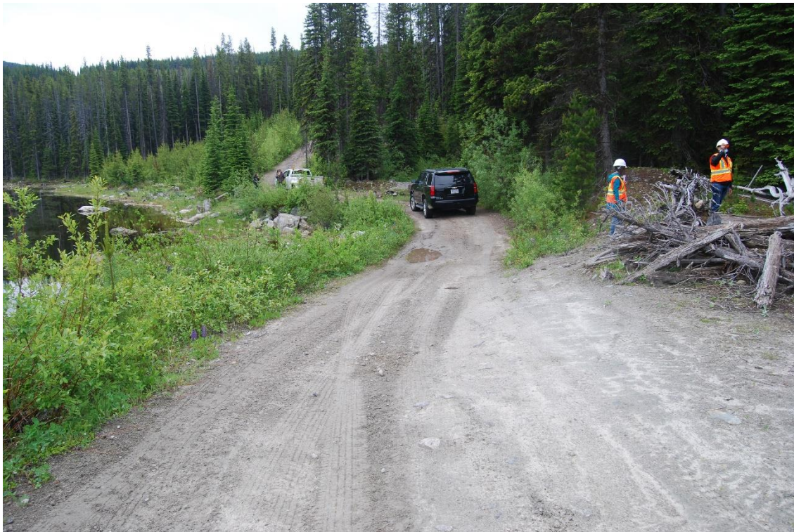
Photo A12: Big Meadow Lake Dam Low Crest Area close to Left Abutment
