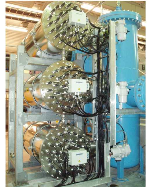
Ultraviolet Light Reactors at the Treatment Plant
