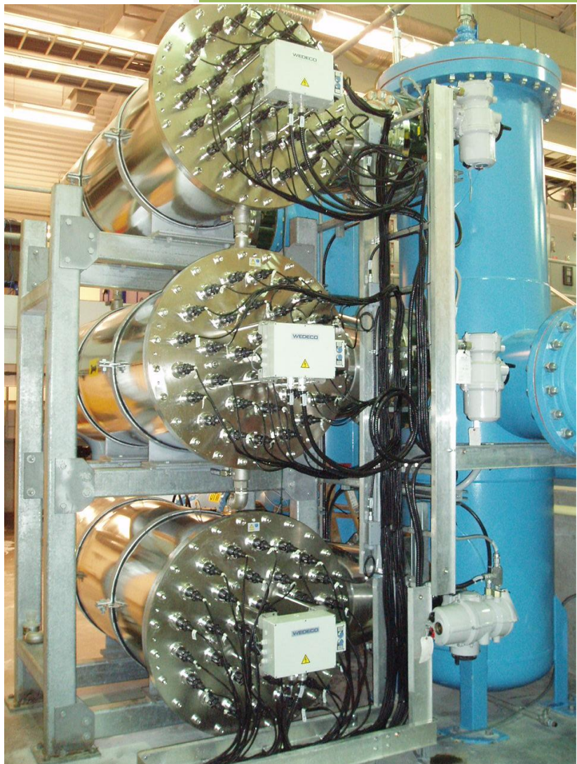
Naramata Water Treatment Plant – UV Disinfection Vessels
