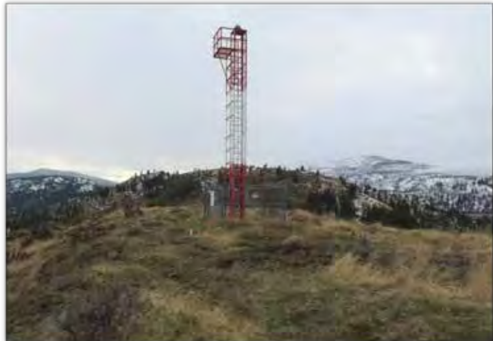
Picture 1: Kaleden E911 Radio Communications Site
