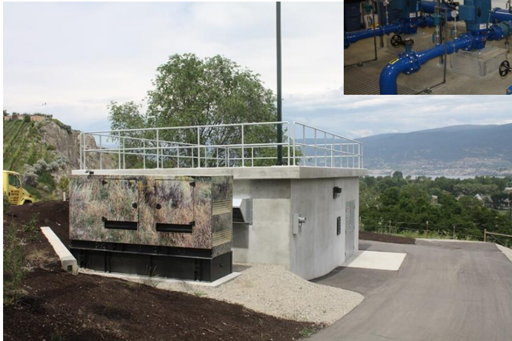
Photo 5 - 6: West Bench pump station and interior showing pumps
