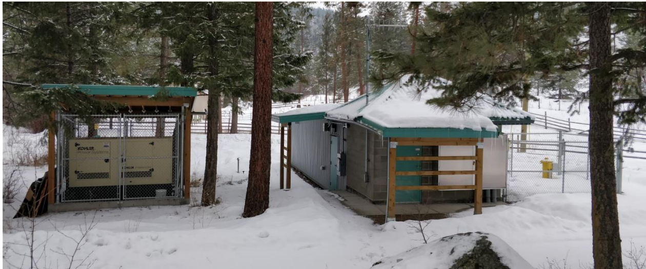
Photo 12: Pump house, uranium treatment and back-up power generation at new plant
