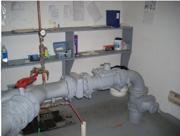
Photo 7: Inside Sage Mesa Pump House
