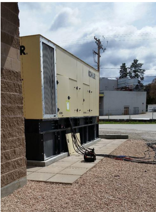
Figure 1. Raw water pump station Generator
