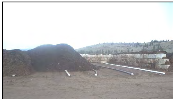
Exhibit 6- 5: Typical ASP system with above-ground piping. Block walls are used to separate batches and better utilize available space.
