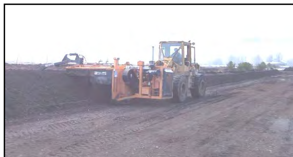
Exhibit 6- 4: Typical windrow operation with a specialized turner mounted on a front-end loader.
