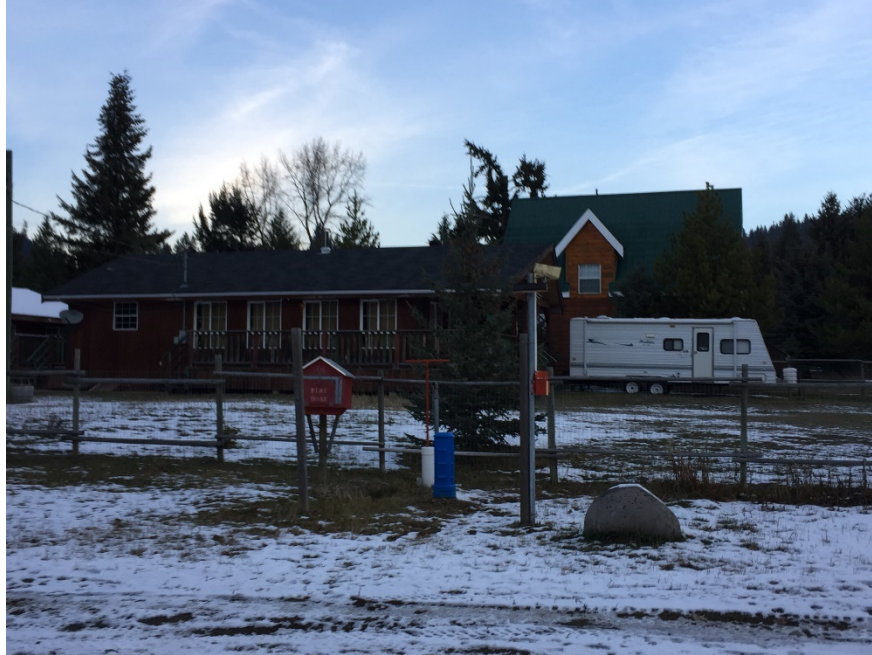
Figure 13 One of a number of standpipes equipped with a hose box and warning alarm located throughout the Missezula Lake community.
